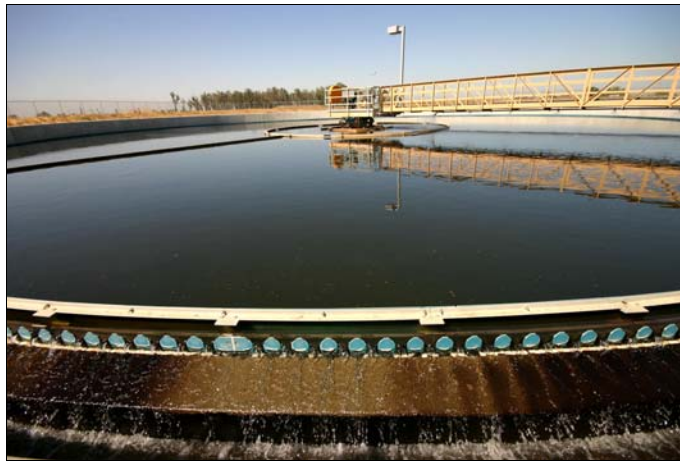
The City must upgrade the wastewater treatment plant to meet new state and federal water quality standards.
