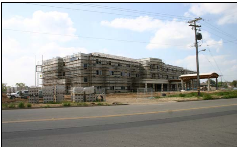
New Marriott Courtyard under construction on Motel Drive. Over the past year, interest in lodging investment in Merced has increased dramatically.
